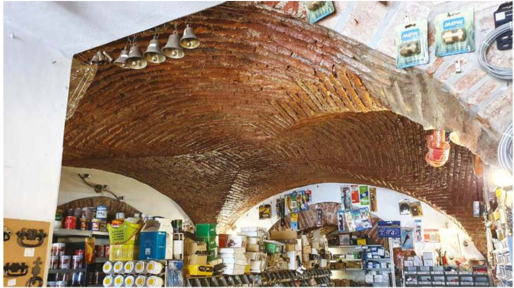
Fig. 5 Borba. Rua Marquês de Marialva 19. Four different ceiling structures in the same ground floor. The second and third compartments are covered by groin vaults; the front compartment shares an almost flat though timbrel vault, and timbrel vaults combined with metallic beams; and the side corridor displays a barrel vault. Source: author, 2024.
