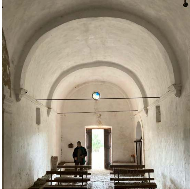
Fig. 9 Barrel vaults in ground-floor functional spaces. Cellar in Monte da Balsa, Portel. Source: authors, 2023.
