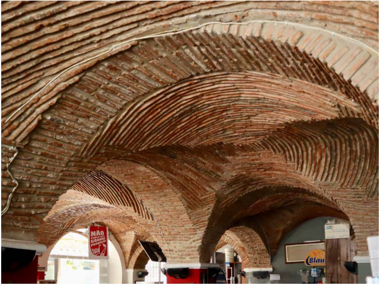
Fig. 5 Vault with bricks assembled perpendicularly to the intrados. Shop in Rua Cons. Augusto de Castro 11, Moura. Source: authors, 2023.
