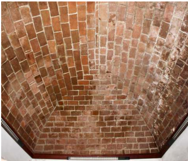
Fig. 6 Vault with bricks assembled horizontally/tangentially to the intrados (timbel vault). House in Rua das Manhãs, Alvito. Source: authors, 2023.
