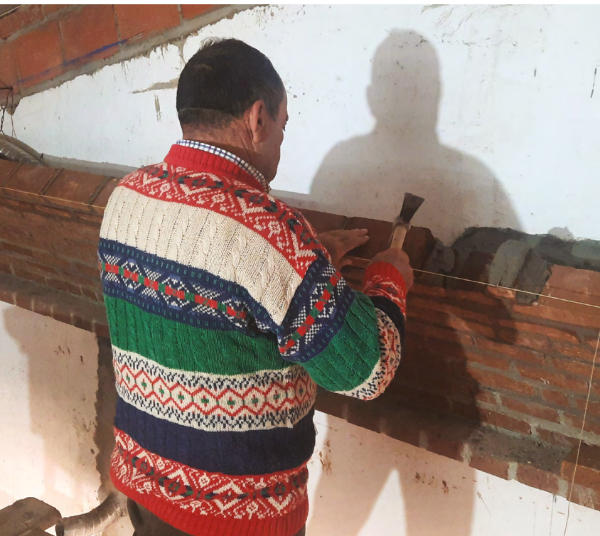
Fig. 2 A master builder at work during the construction of a vault in Baleizão. Source: Mafalda Batista Pacheco, 2023.
